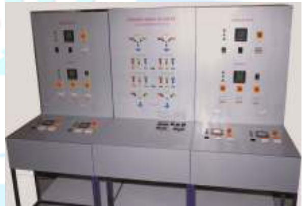
Image 1: SCADA hardware components connected to the model with provision for 3 generators, 3 loads and 3 transmission lines
